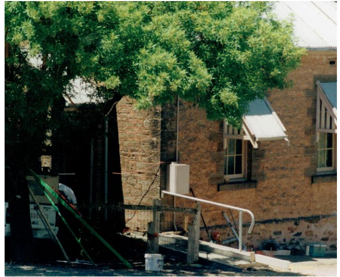
An access ramp under construction for western porch doorway. At the foot of the ramp the after-hours book receival container was installed. Photo National Trust, Tidy Town collection.
